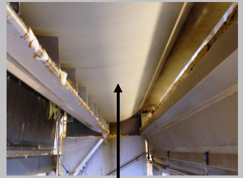
Under the dry roller the new cleaning equipment is placed with the sanding head from Flex Trim, which sands the roller clean for dried layer of potato mash.
